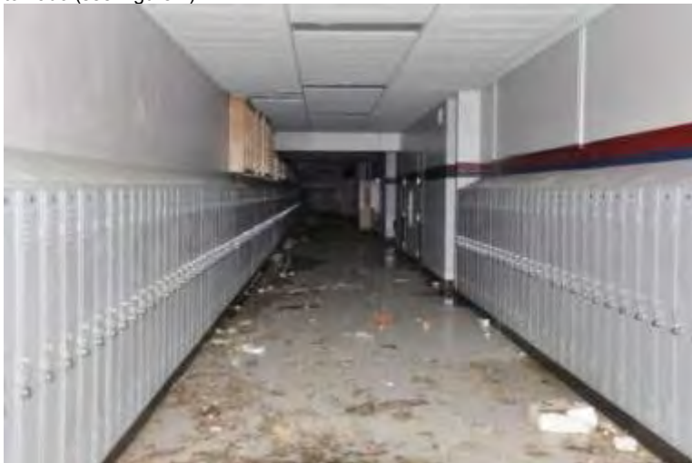
Figure 2 (Figure 6-52 of the MAT Report): View of a corridor designated as a tornado refuge area in Joplin High School. The debris was blown into the corridor during the tornado.
