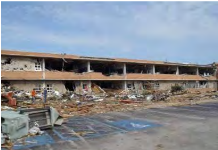
Figure 4 (Figure 6-53 of the MAT Report): North classroom wing damage of Joplin High School.
