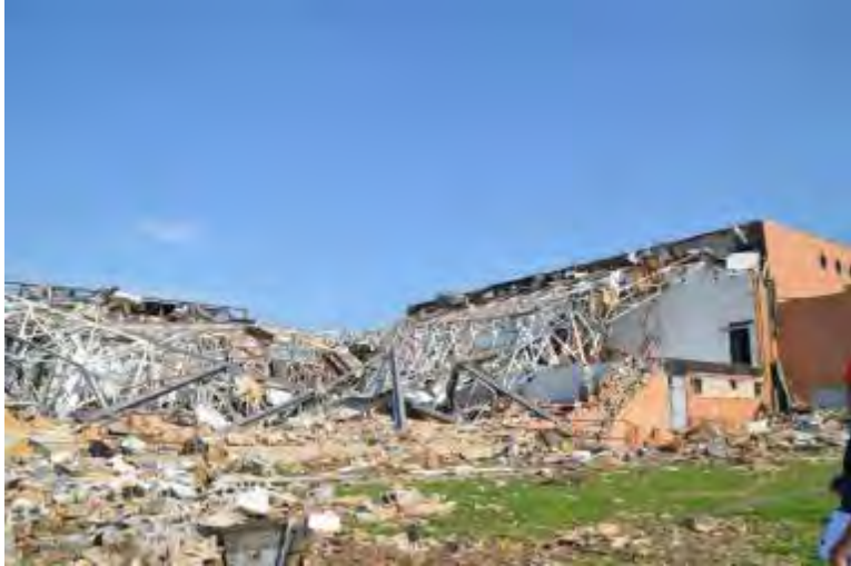
Figure 3 (Figure 6-56): View of the collapsed primary gymnasium of Joplin High School. The gymnasium collapsed through progressive failure.
