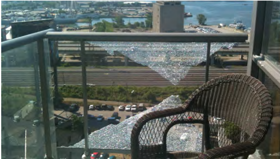
July 2012 - Broken tempered glass assembly 15th floor condo at 33 Mill Street, in Toronto.
